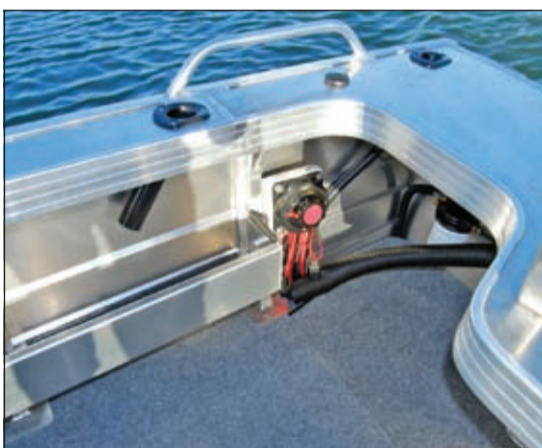
Battery isolation switch.
